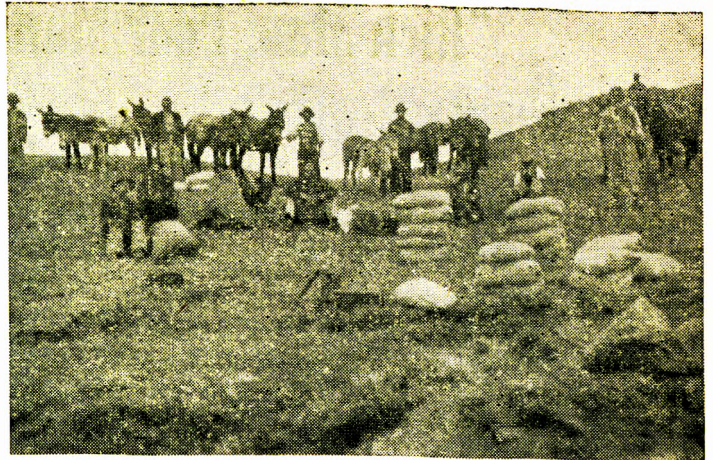
Scene near Cohoni, Bolivia. Sacks of cement, a tile machine, and other equipment for use in the construction of a chapel.
